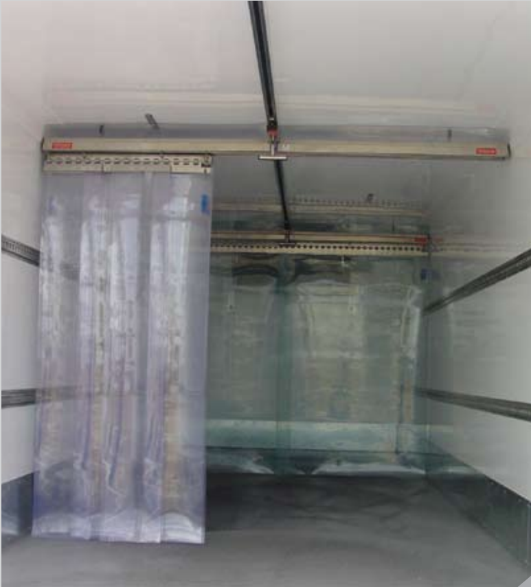
Twin gliding truck systems fitted on a central track allows multiple temperature zones freezer, chiller and dry goods
