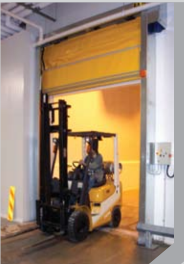
Induction loops activating rapid door
